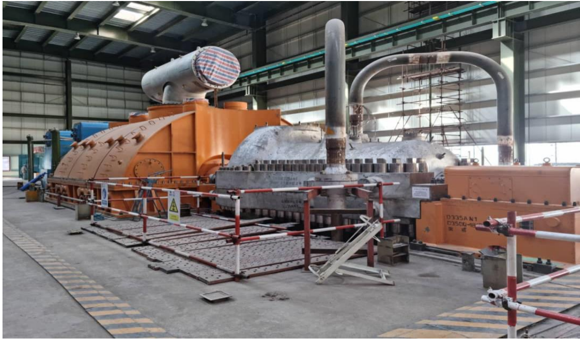
Hwange 7 & 8 Expansion project: Generator number 7
